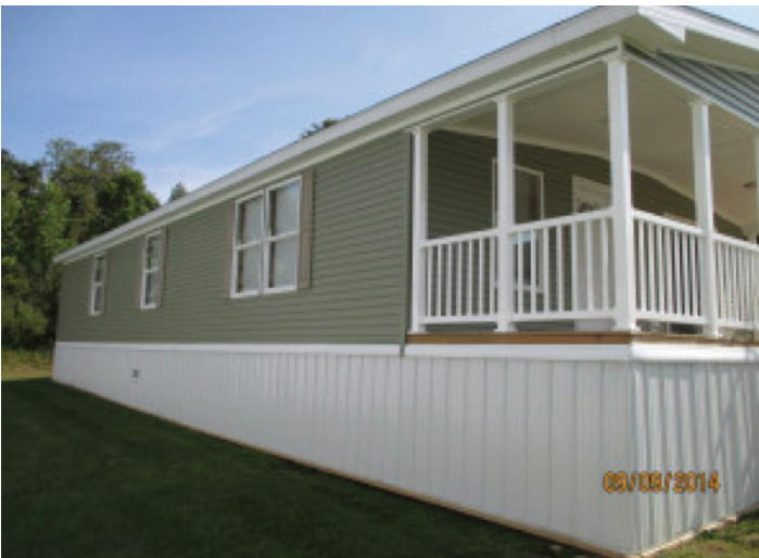
Water gets captured inside skirting.
