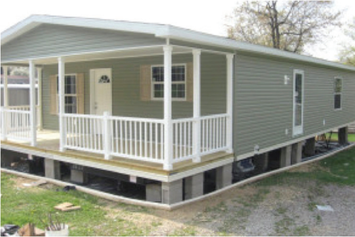
Home sits in a "pit" No way for water to escape.
