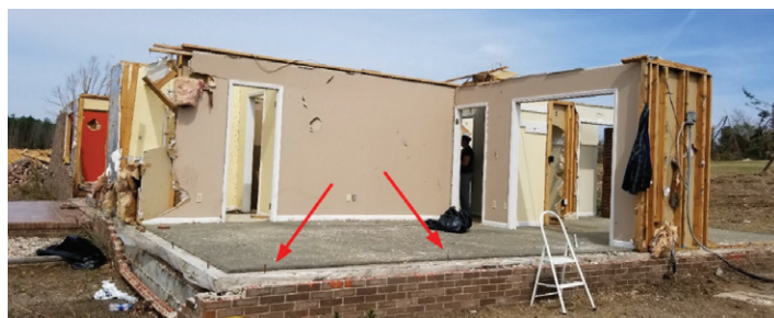
Slab-on-grade foundation anchor bolts with no nuts installed to secure the sill plate to the slab (Lee County, Alabama - March 2019).
