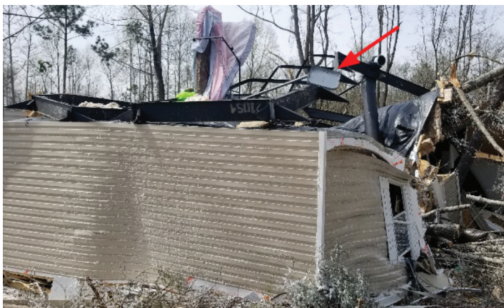
Surface mount pan anchor still attached to home frame (Lee County, Alabama - March 2019).
